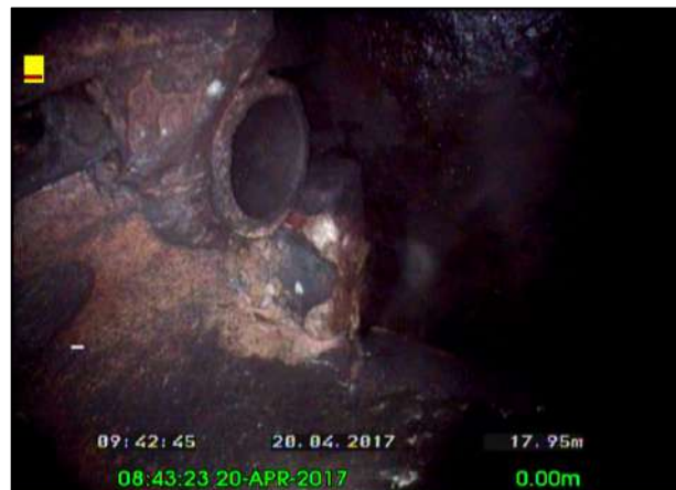
Photo: 33_33_200_A.jpg, 00:06:54 17.95m, Connection other than junction, at 10 o'clock, diameter 150mm
