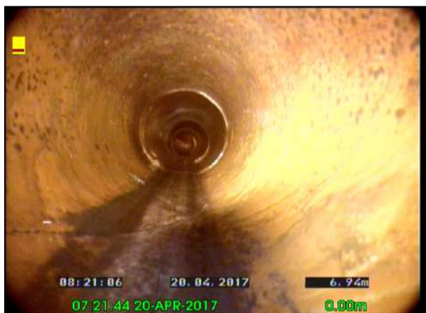
Photo: 35_35_221_A.jpg, 00:04:10 6.93m, Crack, longitudinal, at 7 o'clock
