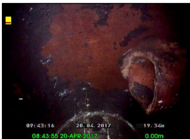
Photo: 33_33_201_A.jpg, 00:07:25 19.34m, Connection other than junction, at 2 o'clock, diameter 150mm
