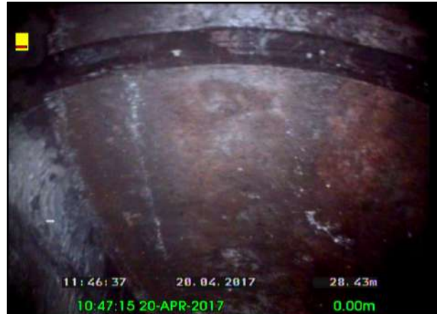
Photo: 41_41_272_A.jpg, 00:08:44 28.43m, Open joint, medium
