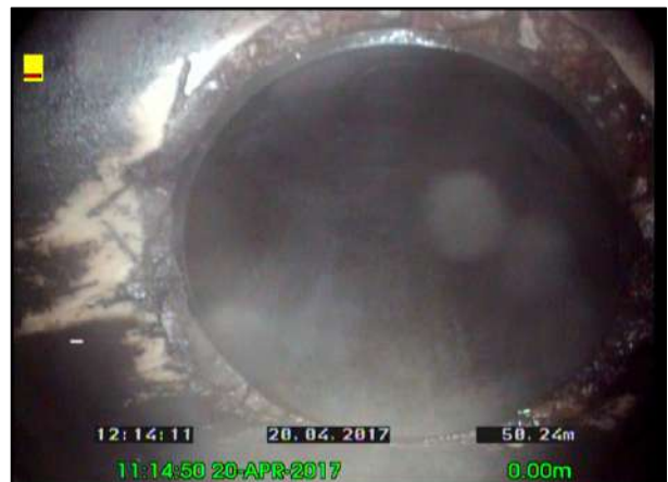
Photo: 39_39_252_A.jpg, 00:09:29 50.24m, Connection other than junction, at 12 o'clock, diameter 150mm
