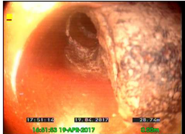
Photo: 20_20_123_A.jpg, 00:09:06 28.74m, Connection other than junction, at 2 o'clock, diameter 100mm
