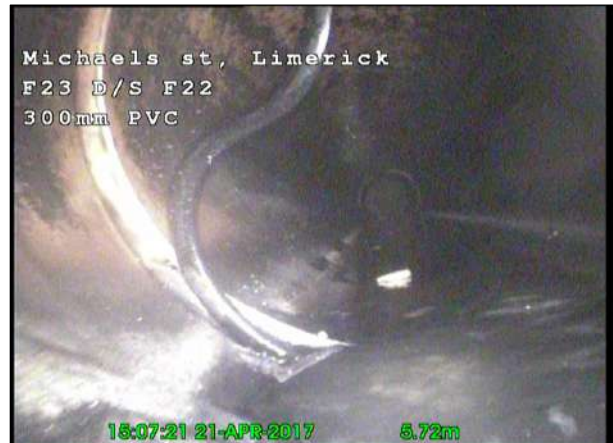
Photo: 47_47_306_A.jpg, 00:00:22 5.72m, Sealing ring intruding, from 6 to 12 o'clock
