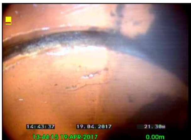
Photo: 16_16_75_A.jpg, 00:13:35 21.38m, Open joint, medium
