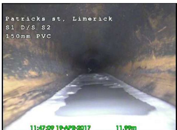
Photo: 31_31_182_A.jpg, 00:01:40 11.99m, Water level, 10% of the vertical dimension Remarks: DIP IN LINE
