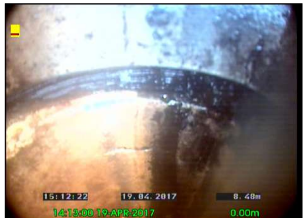
Photo: 17_17_90_A.jpg, 00:05:21 8.48m, Open joint, medium
