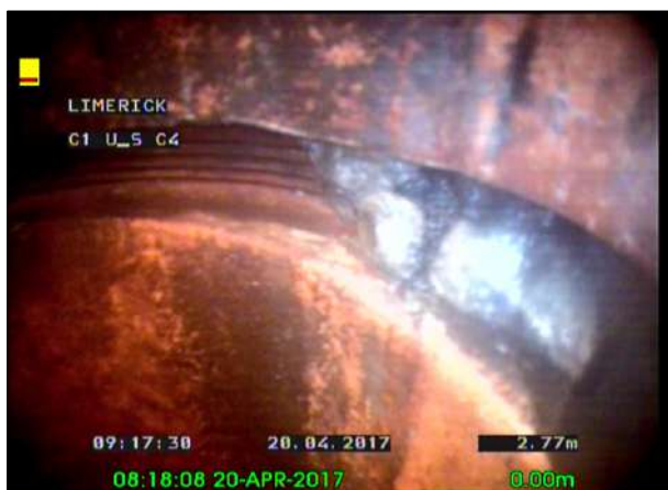
Photo: 34_34_210_A.jpg, 00:02:02 2.77m, Open joint, medium
