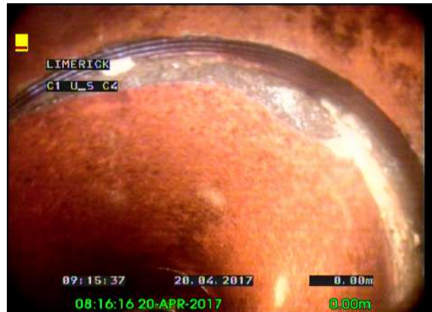
Photo: 34_34_207_A.jpg, 00:00:09 0m, Open joint, medium
