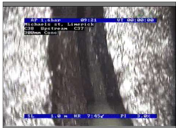
Photo: 8_8_36_A.jpg, 00:00:27 1m, Open joint, medium
