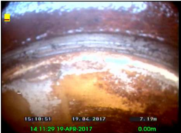
Photo: 17_17_87_A.jpg, 00:03:50 7.19m, Open joint, medium
