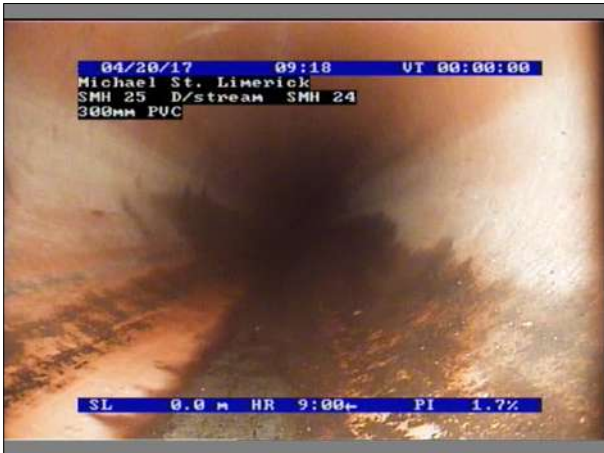
Photo: 1_1_1_A.jpg, 00:00:00 0m, Start node type, manhole, reference number : SMH 25
