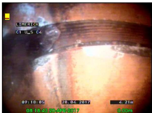
Photo: 34_34_211_A.jpg, 00:02:37 4.21m, Open joint, medium
