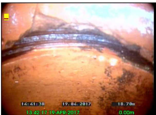
Photo: 16_16_71_A.jpg, 00:11:36 18.78m, Open joint, medium
