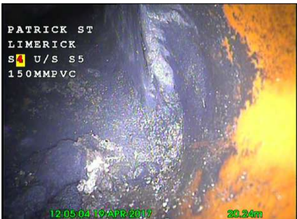
Photo: 27_27_161_A.jpg, 00:05:12 20.24m, Start node type, manhole, reference number : SMH 4
