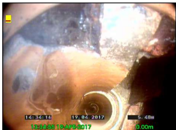
Photo: 16_16_61_A.jpg, 00:04:14 5.48m, Broken pipe, from 6 to 9 o'clock Remarks: IN CHAMBER
