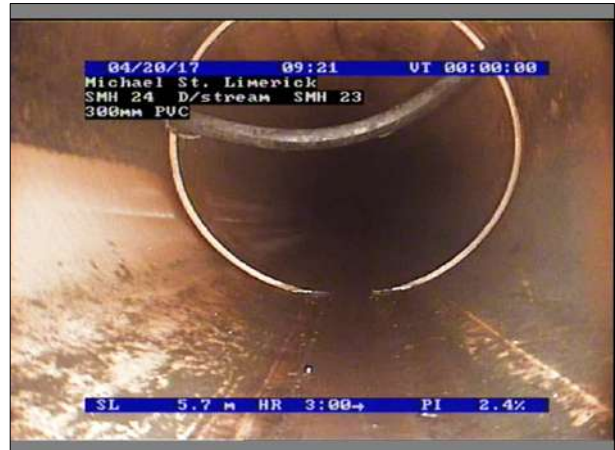
Photo: 3_3_21_A.jpg, 00:00:50 5.7m, Sealing ring intruding, from 9 to 2 o'clock
