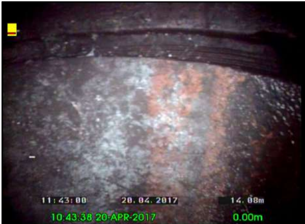
Photo: 41_41_267_A.jpg, 00:05:07 14.08m, Open joint, medium
