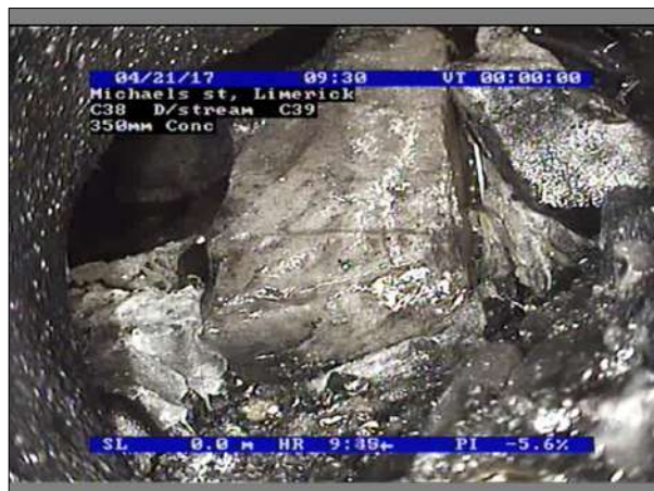
Photo: 9_9_41_A.jpg, 00:00:02 0m, Other obstacles, brick or masonry in invert, from 12 to 12 o'clock, 95% cross-sectional area loss Remarks: pipe fully blocked. possibly collapsed, unable to determine
