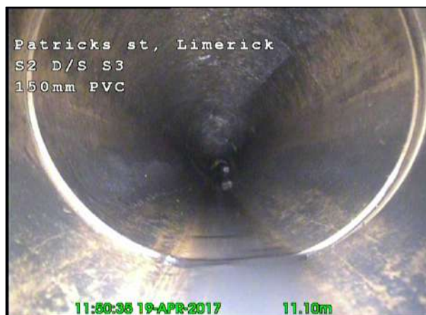
Photo: 32_32_188_A.jpg, 00:01:39 11.1m, Open joint, medium
