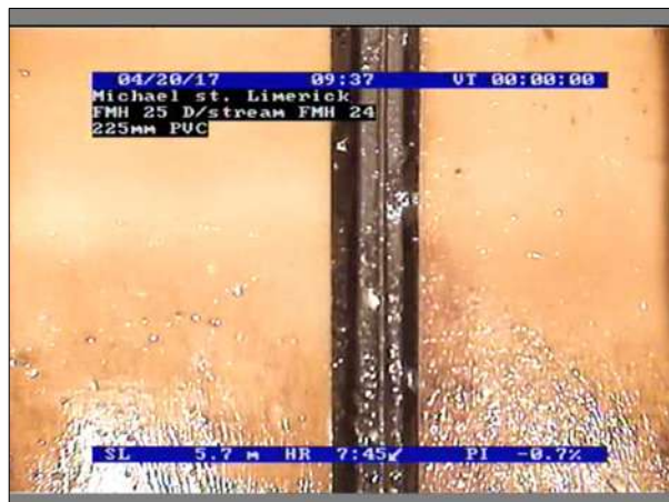
Photo: 4_4_26_A.jpg, 00:00:50 5.7m, Open joint, medium
