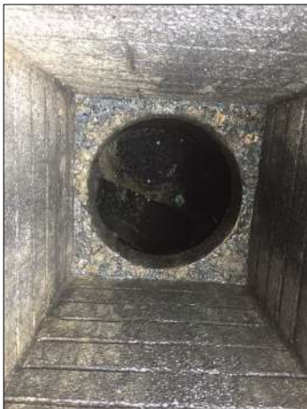
Photo: 2017-04-28-PHOTO-00000052.jpg 9.01m, General photograph taken at this point Remarks: manhole C30 picture
