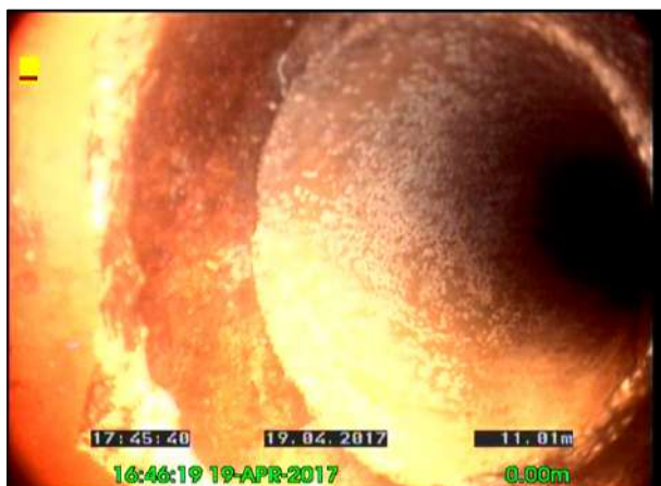
Photo: 20_20_116_A.jpg, 00:03:32 11.01m, Connection other than junction, at 2 o'clock, diameter 100mm
