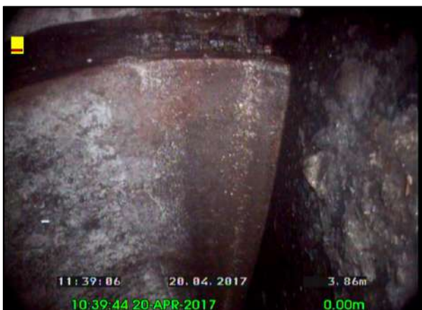
Photo: 41_41_261_A.jpg, 00:01:13 3.86m, Open joint, medium
