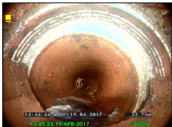
Photo: 16_16_79_A.jpg, 00:14:42 22.75m, Joint displaced, large Remarks: LEAVING CHAMBER TO LINE
