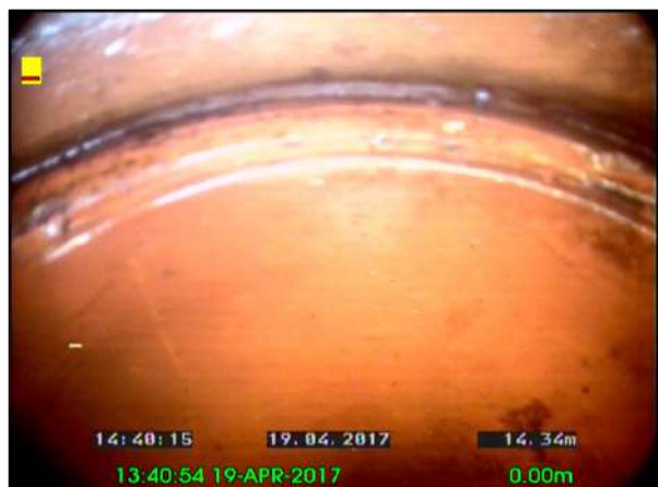
Photo: 16_16_70_A.jpg, 00:10:13 14.34m, Open joint, medium
