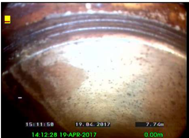
Photo: 17_17_89_A.jpg, 00:04:49 7.74m, Open joint, medium
