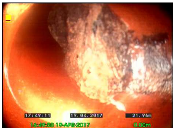
Photo: 20_20_119_A.jpg, 00:06:09 20.79m, Connection other than junction, at 12 o'clock, diameter 100mm
