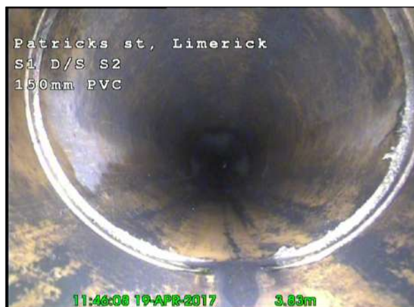
Photo: 31_31_181_A.jpg, 00:00:39 3.83m, Open joint, medium
