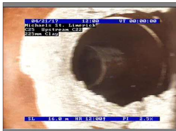
Photo: 12_12_52_A.jpg, 00:03:38 16m, Connection other than junction, at 12 o'clock, diameter 100mm
