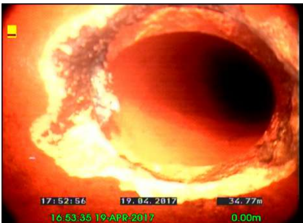
Photo: 20_20_125_A.jpg, 00:10:49 34.77m, Connection other than junction, at 2 o'clock, diameter 100mm
