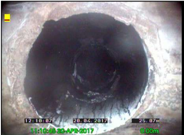
Photo: 39_39_249_A.jpg, 00:05:24 25.87m, Connection other than junction, at 12 o'clock, diameter 225mm
