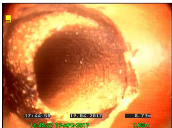
Photo: 20_20_115_A.jpg, 00:02:50 8.73m, Connection other than junction, at 10 o'clock, diameter 100mm
