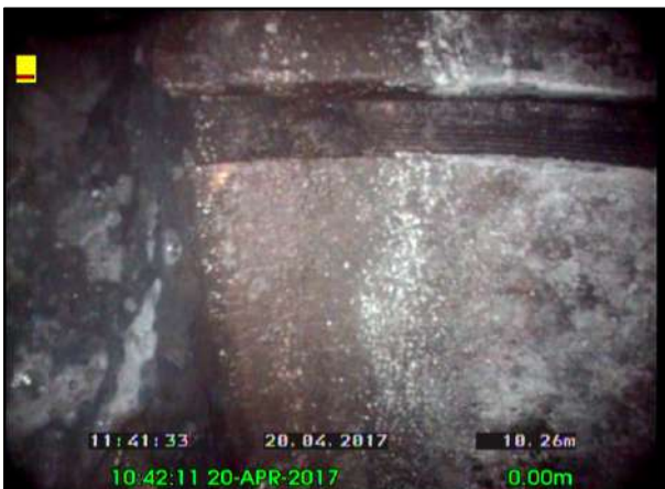
Photo: 41_41_265_A.jpg, 00:03:40 10.26m, Open joint, medium
