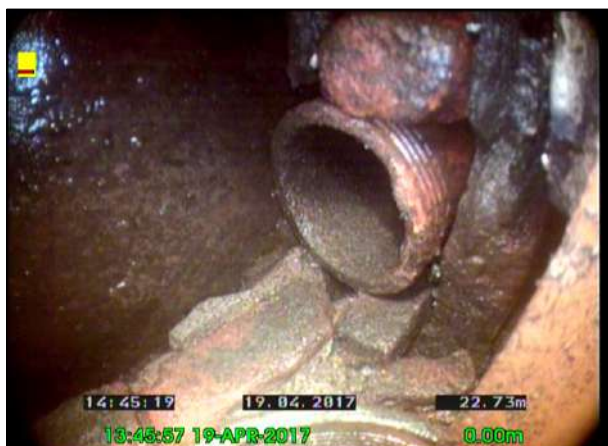
Photo: 16_16_77_A.jpg, 00:14:19 22.68m, Connection other than junction, at 3 o'clock, diameter 150mm
