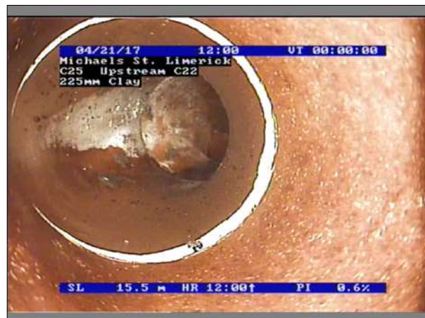
Photo: 12_12_50_A.jpg, 00:03:03 15.5m, Connection other than junction, at 12 o'clock, diameter 100mm
