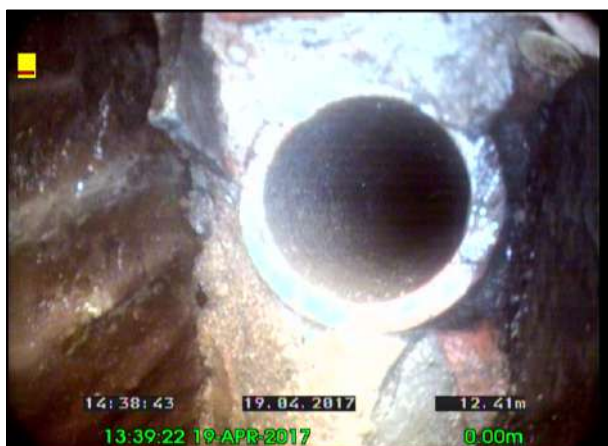
Photo: 16_16_67_A.jpg, 00:08:41 12.41m, Connection other than junction, at 3 o'clock, diameter 100mm
