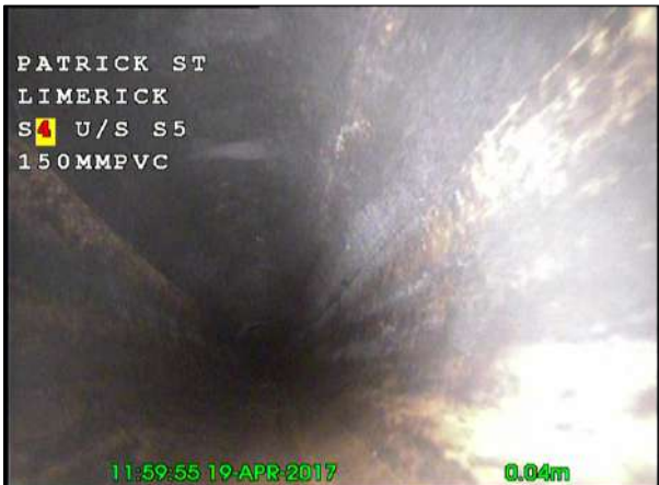
Photo: 27_27_158_A.jpg, 00:00:02 0m, Start node type, manhole, reference number : SMH 4
