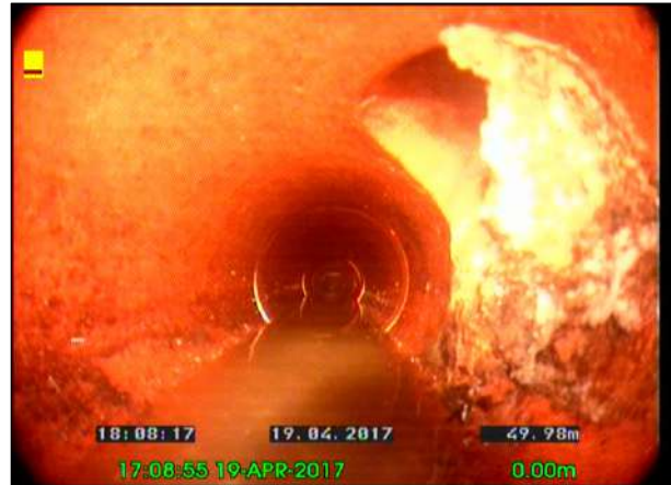
Photo: 21_21_134_A.jpg, 00:09:31 49.98m, General photograph taken at this point Remarks: OF CONNECTION
