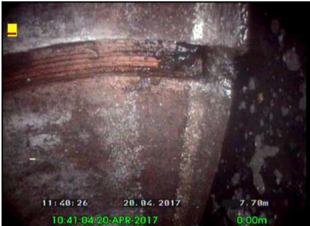
Photo: 41_41_263_A.jpg, 00:02:33 7.78m, Open joint, medium
