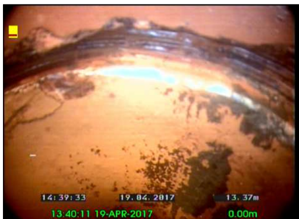
Photo: 16_16_69_A.jpg, 00:09:31 13.37m, Open joint, medium
