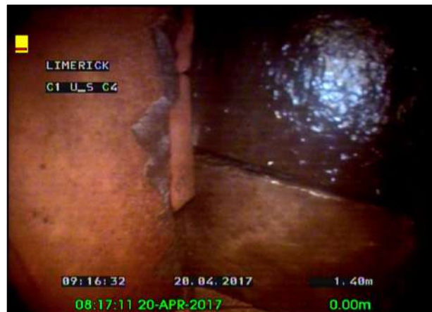
Photo: 34_34_209_A.jpg, 00:00:55 1.4m, Broken pipe, from 10 to 2 o'clock Remarks: TOP OF PIPE MISSING AND CAPPED OVER
