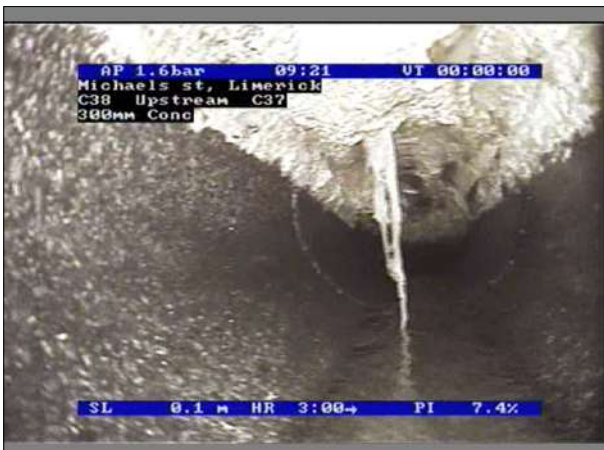
Photo: 8_8_35_A.jpg, 00:00:17 0.1m, Attached deposits, grease, from 10 to 2 o'clock, 10% cross-sectional area loss Remarks: Jet unable to remove,
