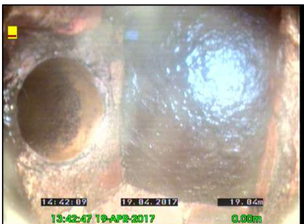
Photo: 16_16_73_A.jpg, 00:12:07 19.04m, Connection other than junction, at 11 o'clock, diameter 150mm
