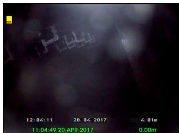
Photo: 39_39_246_A.jpg, 00:01:18 4.01m, General remark Remarks: INTERMEDIATE BURIED MANHOLE ON LINE
