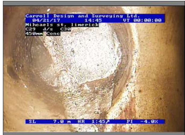
Photo: 15_15_321_A.jpg, 00:01:21 7m, Connection other than junction, closed, at 2 o'clock, diameter 150mm
