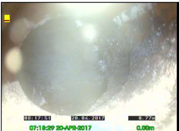
Photo: 35_35_217_A.jpg, 00:00:55 0.77m, Connection other than junction, at 12 o'clock, diameter 150mm
