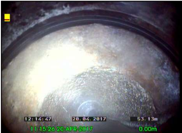
Photo: 39_39_253_A.jpg, 00:10:04 53.13m, Open joint, medium
