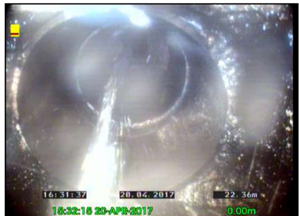
Photo: 38_38_240_A.jpg, 00:03:09 22.36m, Connection other than junction, at 12 o'clock, diameter 150mm
