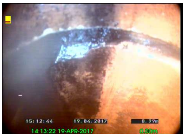
Photo: 17_17_91_A.jpg, 00:05:50 8.99m, Open joint, medium
