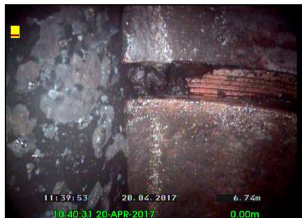
Photo: 41_41_262_A.jpg, 00:02:00 6.74m, Open joint, medium
