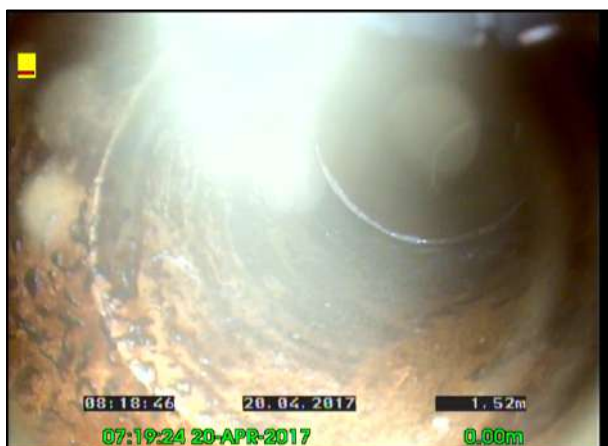
Photo: 35_35_219_A.jpg, 00:01:49 1.52m, Connection other than junction, at 2 o'clock, diameter 150mm
