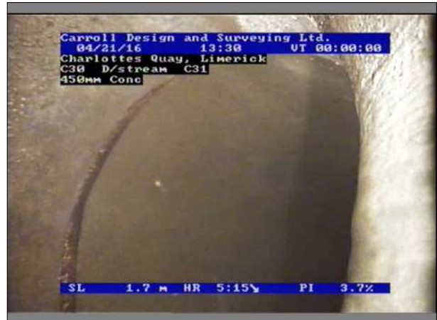
Photo: 13_13_314_A.jpg, 00:00:44 1.7m, Connection other than junction, at 6 o'clock, diameter 450mm Remarks: backdrop
