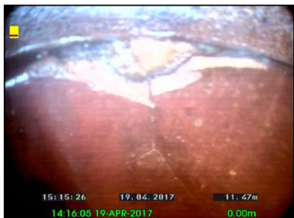
Photo: 17_17_96_A.jpg, 00:08:26 11.47m, Broken pipe, at 10 o'clock
