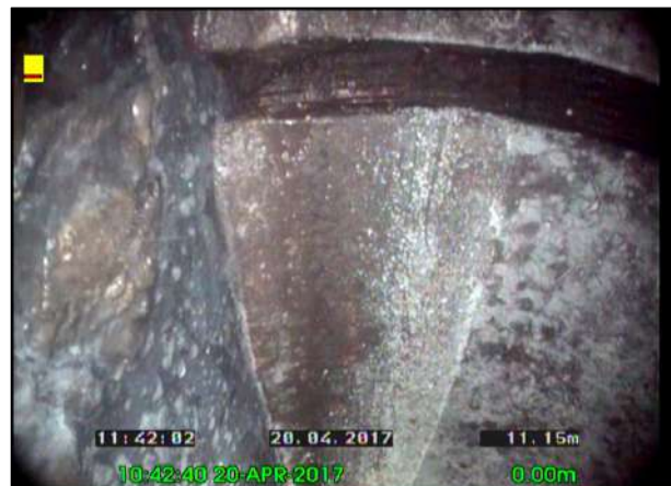
Photo: 41_41_266_A.jpg, 00:04:09 11.15m, Open joint, medium
