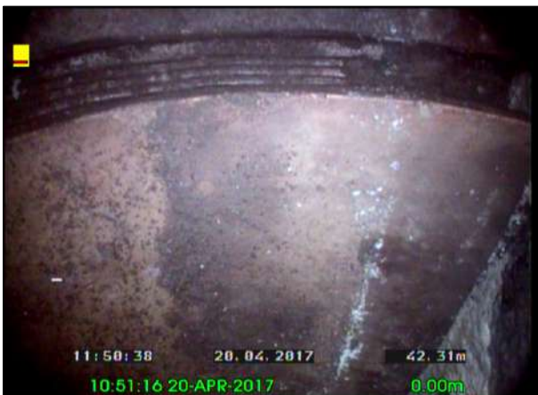
Photo: 41_41_278_A.jpg, 00:12:46 42.31m, Open joint, medium
