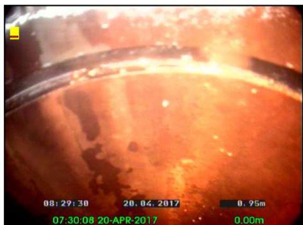
Photo: 36_36_227_A.jpg, 00:00:29 0.95m, Open joint, medium
