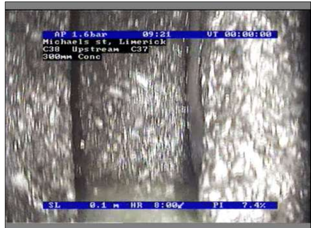
Photo: 8_8_34_A.jpg, 00:00:10 0.1m, Open joint, medium
