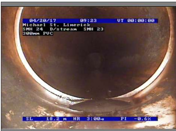
Photo: 3_3_22_A.jpg, 00:02:32 18.2m, Open joint, medium
