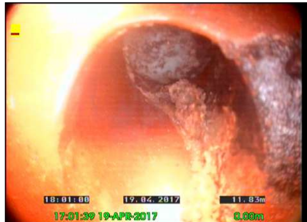
Photo: 21_21_130_A.jpg, 00:02:15 11.83m, Connection other than junction, at 2 o'clock, diameter 100mm
