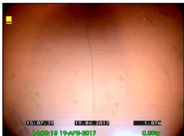
Photo: 17_17_84_A.jpg, 00:00:38 1.07m, Crack, longitudinal, at 6 o'clock
