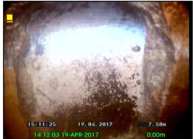
Photo: 17_17_88_A.jpg, 00:04:24 7.5m, Hole in drain/ sewer, at 12 o'clock
