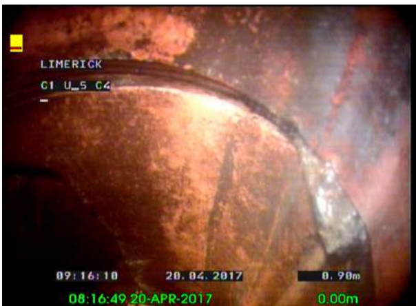
Photo: 34_34_208_A.jpg, 00:00:42 0.9m, Open joint, medium
