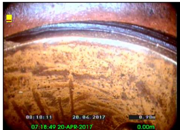
Photo: 35_35_218_A.jpg, 00:01:15 0.98m, Open joint, medium
