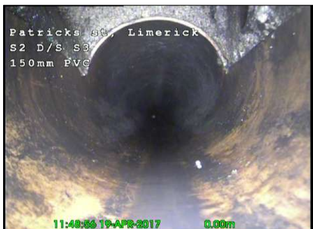
Photo: 32_32_186_A.jpg, 00:00:01 0m, Start node type, manhole, reference number : SMH 2
