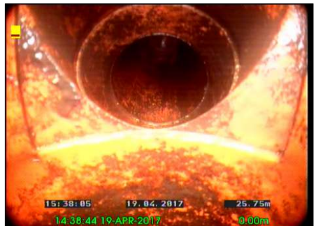
Photo: 18_18_104_A.jpg, 00:03:52 25.75m, Connection other than junction, at 12 o'clock, diameter 150mm
