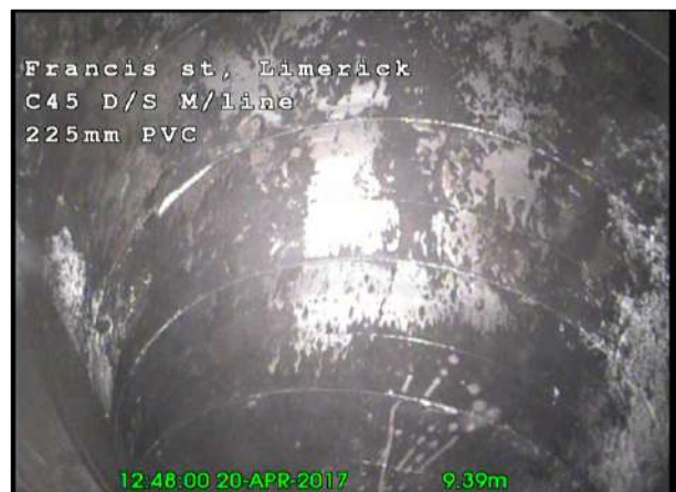
Photo: 43_43_288_A.jpg, 00:01:22 9.39m, Line deviates down Remarks: DOWNWARDS INTO MAINLINE
