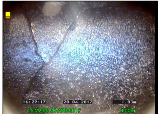
Photo: 38_38_238_A.jpg, 00:00:32 1.83m, Cracks, multiple, from 5 to 12 o'clock
