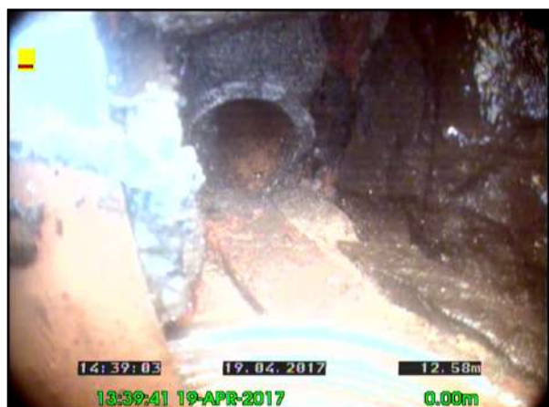
Photo: 16_16_68_A.jpg, 00:09:01 12.58m, Connection other than junction, at 10 o'clock, diameter 100mm
