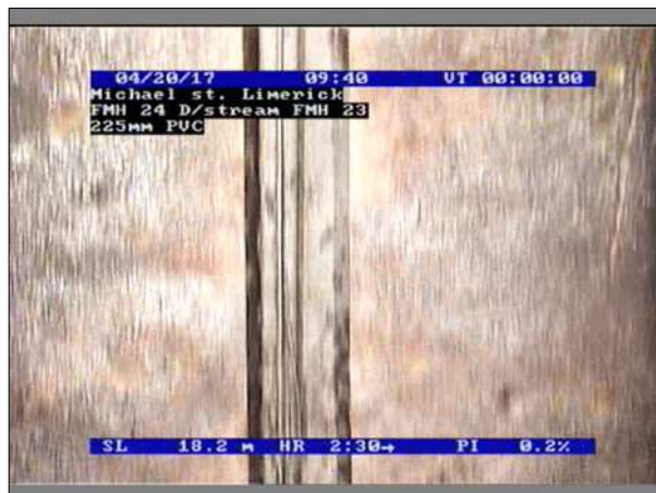
Photo: 5_5_30_A.jpg, 00:02:12 18.2m, Open joint, medium
