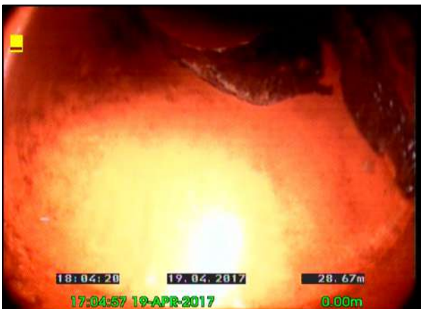
Photo: 21_21_131_A.jpg, 00:05:34 28.67m, Connection other than junction, at 2 o'clock, diameter 100mm
