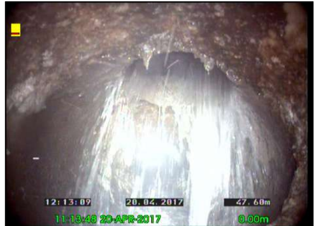
Photo: 39_39_250_A.jpg, 00:08:27 47.6m, Connection other than junction, at 12 o'clock, diameter 150mm
