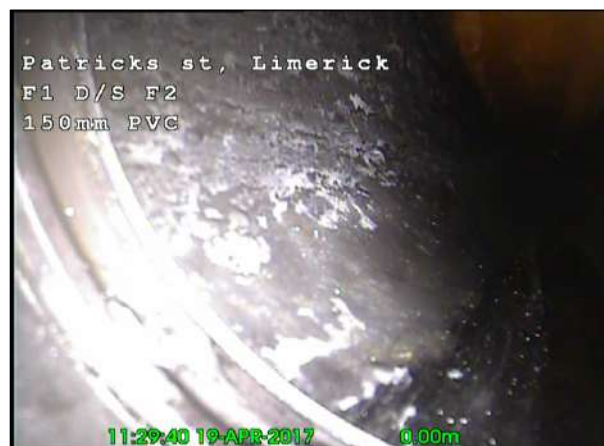
Photo: 28_28_164_A.jpg, 00:00:07 0.1m, Open joint, medium
