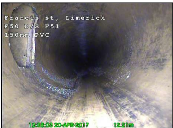
Photo: 44_44_293_A.jpg, 00:01:36 12.21m, Connection other than junction, at 9 o'clock, diameter 100mm
