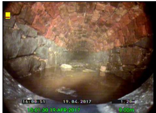
Photo: 19_19_109_A.jpg, 00:00:37 1.2m, Start node type, major connection without manhole, reference number : C 7 Remarks: connecting to mainline culvert
