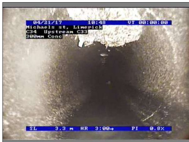
Photo: 11_11_45_A.jpg, 00:00:21 3.3m, Attached deposits, fouling, from 12 to 2 o'clock, 5% cross-sectional area loss
