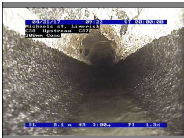
Photo: 8.8_38_A.jpg, 00:01:44 8.1m, Attached deposits, grease, from 10 to 2 o'clock, 10% cross-sectional area loss Remarks: continuous
