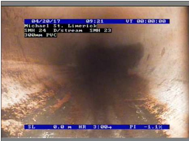
Photo: 3_3_3_A.jpg, 00:00:00 0m, Start node type, manhole, reference number : SMH 24
