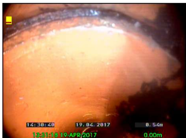
Photo: 16_16_59_A.jpg, 00:00:38 0.33m, Joint displaced, medium
