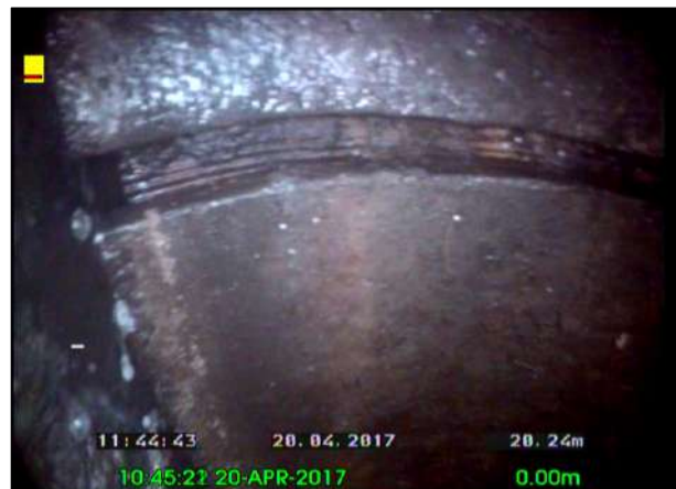
Photo: 41_41_270_A.jpg, 00:06:50 20.24m, Open joint, medium
