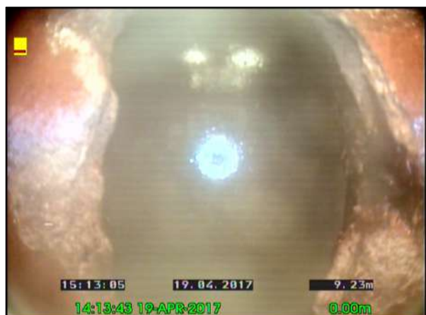
Photo: 17_17_92_A.jpg, 00:06:04 9.22m, Hole in drain/sewer, at 12 o'clock Remarks: COVERED
