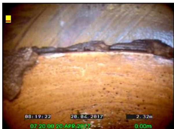
Photo: 35_35_220_A.jpg, 00:02:25 2.32m, Open joint, medium
