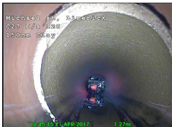
Photo: 46_46_302_A.jpg, 00:00:27 1.27m, Joint displaced, medium
