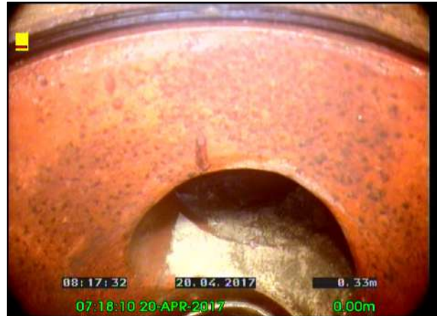
Photo: 35_35_216_A.jpg, 00:00:36 0.33m, Open joint, medium
