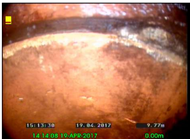
Photo: 17_17_93_A.jpg, 00:06:29 9.76m, Open joint, medium
