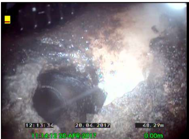
Photo: 39_39_251_A.jpg, 00:08:52 48.3m, Connection other than junction, at 9 o'clock, diameter 150mm
