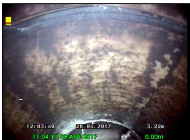
Photo: 39_39_245_A.jpg, 00:00:47 3.22m, Open joint, medium
