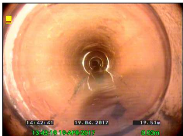
Photo: 16_16_74_A.jpg, 00:12:39 19.51m, Joint displaced, medium
