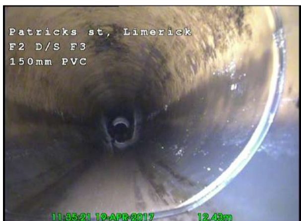
Photo: 29_29_172_A.jpg, 00:01:41 12.43m, Open joint, medium
