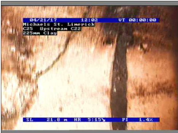
Photo: 12_12_53_A.jpg, 00:05:18 21.8m, Crack, circumferential, from 5 to 10 o'clock
