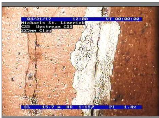
Photo: 12_12_51_A.jpg, 00:03:19 15.7m, Crack, circumferential, from 11 to 2 o'clock
