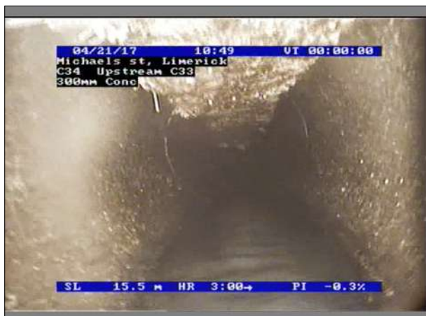
Photo: 11_11_46_A.jpg, 00:01:19 15.5m, Attached deposits, fouling, at 12 o'clock, 5% cross-sectional area loss Remarks: continuous
