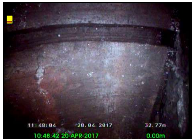
Photo: 41_41_274_A.jpg, 00:10:11 32.77m, Open joint, medium
