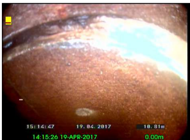
Photo: 17_17_95_A.jpg, 00:07:46 10.8m, Open joint, medium
