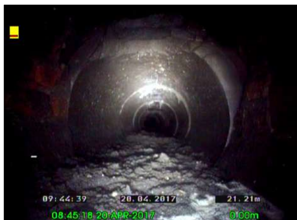
Photo: 33_33_202_A.jpg, 00:08:48 21.21m, Settled deposits, fine, 20% cross-sectional area loss
