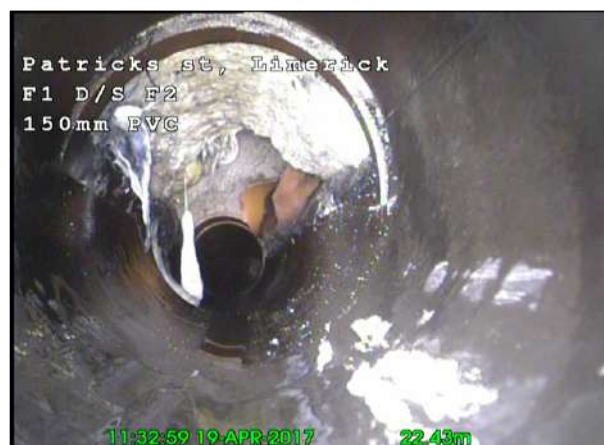
Photo: 28_28_166_A.jpg, 00:03:26 22.43m, Broken pipe, from 9 to 3 o'clock Remarks: COMING INTO MANHOLE
