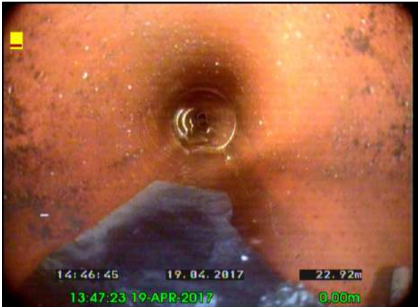
Photo: 16_16_80_A.jpg, 00:16:43 22.92m, Other obstacles, other objects in invert at joint, from 5 to 7 o'clock, 10% cross-sectional area loss Remarks: CAUGHT IN DISPLACED JOINT UNABLE TO REMOVE
