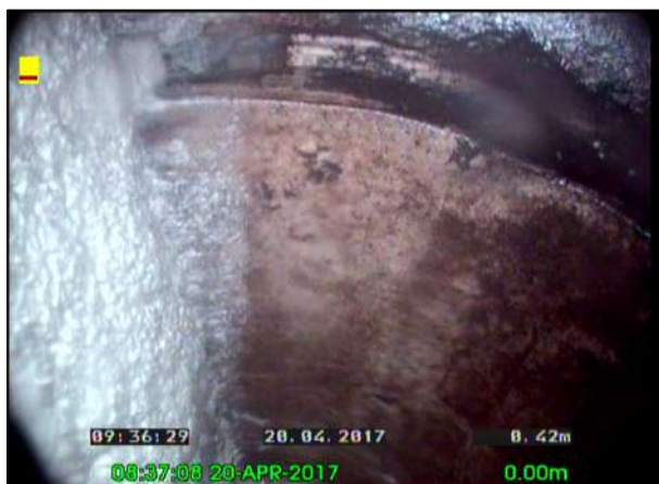
Photo: 33_33_193_A.jpg, 00:00:38 0.42m, Open joint, medium
