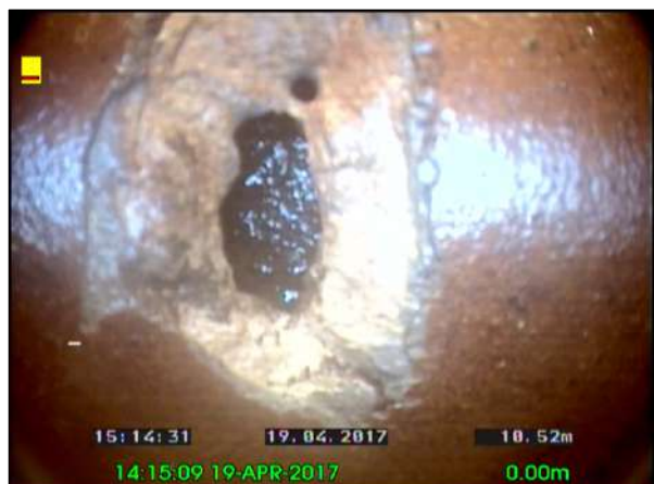
Photo: 17_17_94_A.jpg, 00:07:30 10.52m, Hole in drain/sewer, at 12 o'clock Remarks: HOLE
