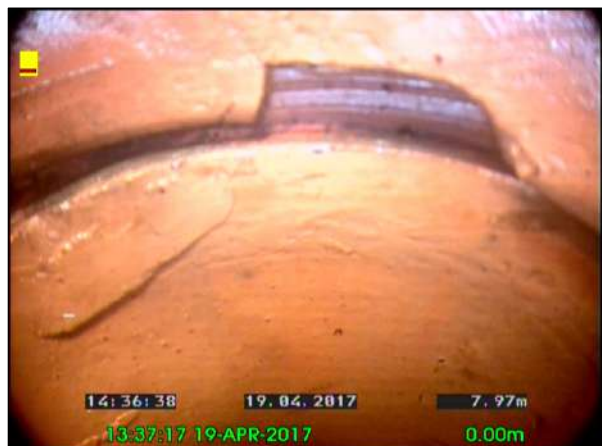
Photo: 16_16_63_A.jpg, 00:06:36 7.97m, Broken pipe, at 1 o'clock
