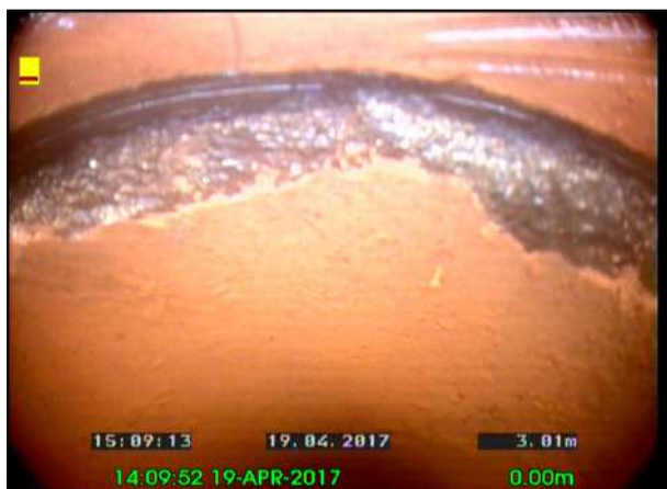
Photo: 17_17_85_A.jpg, 00:02:12 3.01m, Open joint, medium
