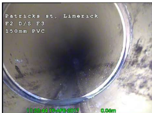
Photo: 29_29_171_A.jpg, 00:00:04 0.1m, Open joint, medium Remarks: SEALING RING INTRUDING AT BOTTOM OF PIPE
